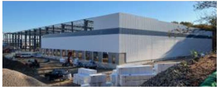
View of the foundation walls for the new building at 35 Saratoga – August 2023
